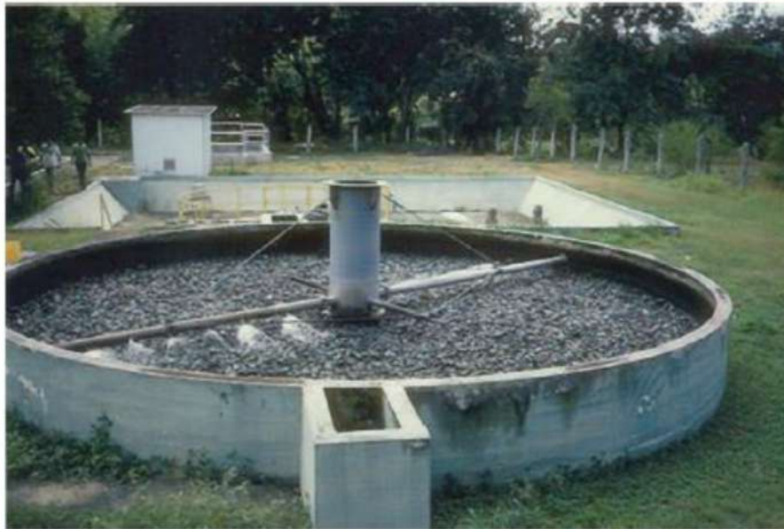
FIGURE 25.7 A trickling filter bed. Here, rocks provide a matrix supporting the growth of a microbial biofilm that actively degrades the organic material in the wastewater under aerobic conditions.
