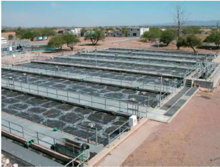
FIGURE 25.8 Secondary treatment: an aeration basin.
