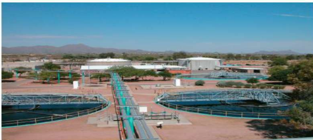
FIGURE 25.6 Three clarifiers (foreground—blue) where suspended organic solids settle out as primary sludge. Also see the two anaerobic sludge digesters in the background (white).
