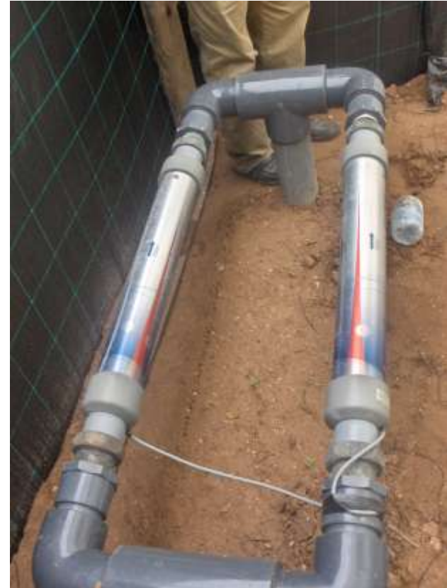
Installation 45 m 3 /h in Morocco
