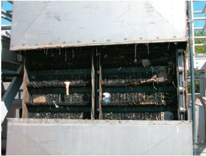
FIGURE 25.4 Removal of large debris from sewage via a “bar screen.”
