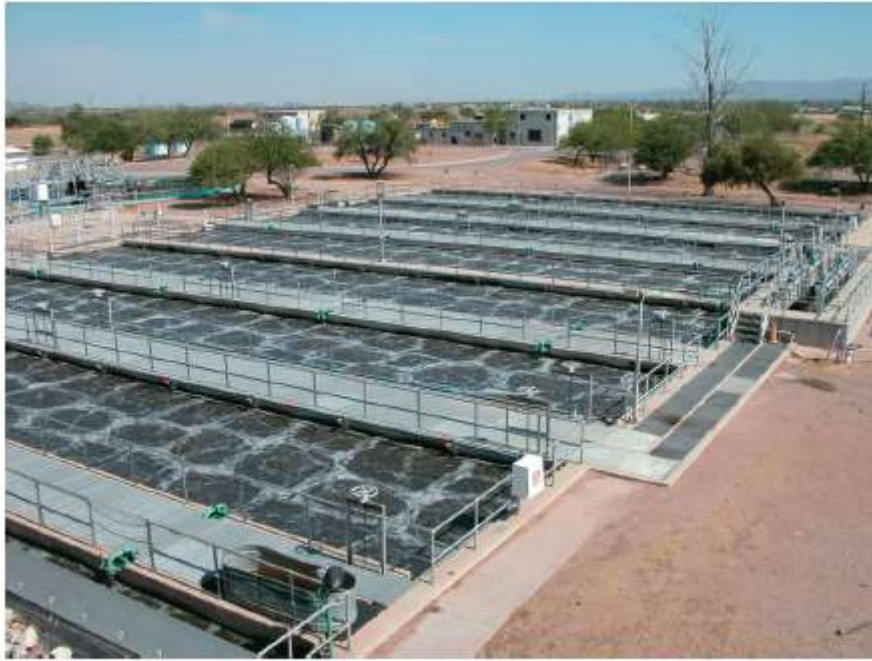
FIGURE 25.8 Secondary treatment: an aeration basin.
